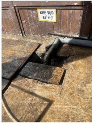
Grease trap area
